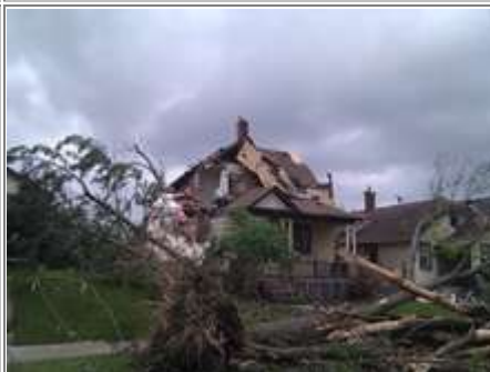
Home damage in Minneapolis, MN
